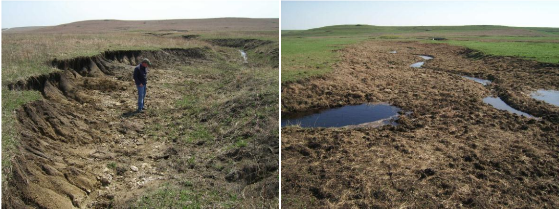
Dry Creek stream channel, before (left) and after restoration construction. View is looking southwest down project area.
